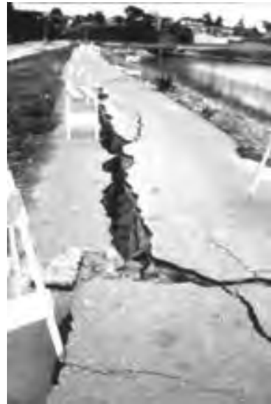
Figure 39 - Lateral Spreading. Loma Prieta Earthquake, October 17, 1989. Lateral spreading damage levee road along the San Lorenzo River.
