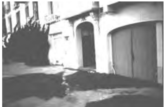
Figure 40 - Loma Prieta Earthquake, October 17, 1989. Lateral spreading, liquefaction and sand boils caused extensive damage in the Marina District of San Francisco, about 60 miles away from the epicenter.
