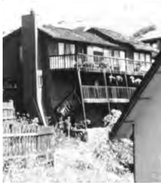
Figure 22 - This hillside home was built on an unbraced tall wall that failed.
